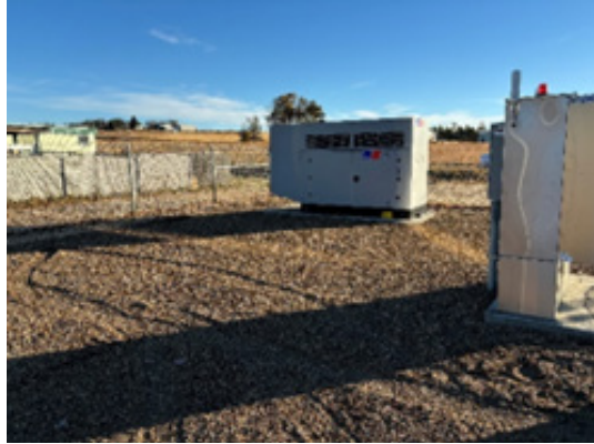
City of Center's generator
