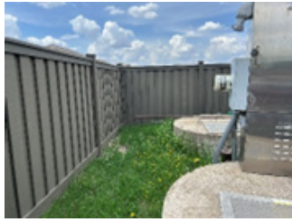
City of Gardner's generator and fence
